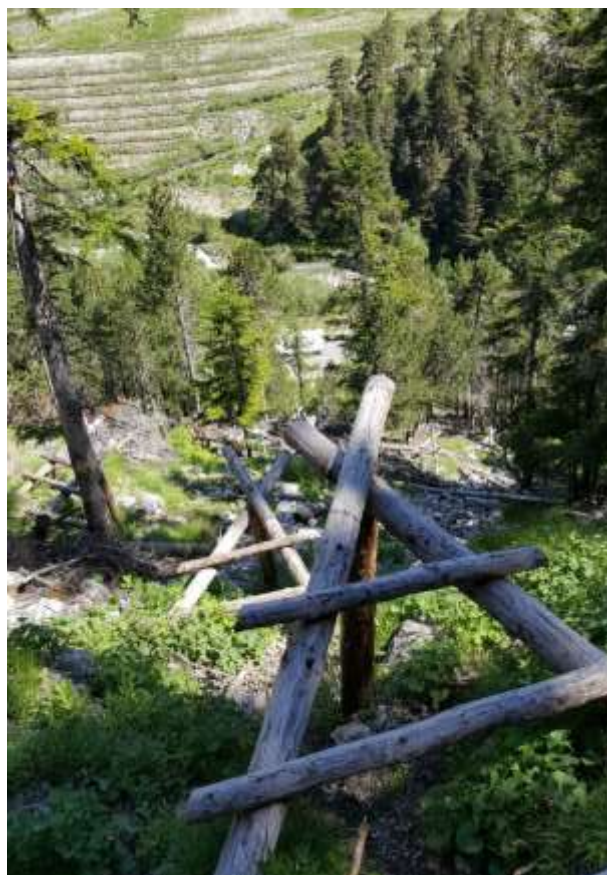
Figure 69: Wooden structures for the reduction of the kinetic energy of rocks along non-forested screes.
